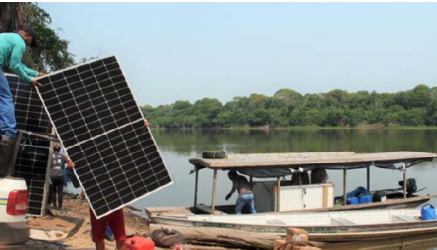
Solar panels arrive at the Rio Pacaás Novos Extractive Reserve in Rondônia, Brazil, to be installed at the local school.
